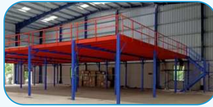
Modular Mezzanine Floor
