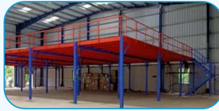
Modular Mezzanine Floor
