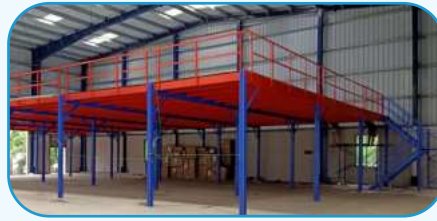
Modular Mezzanine Floor
