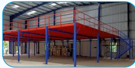
Modular Mezzanine Floor
