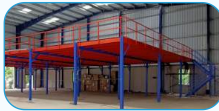
Modular Mezzanine Floor
