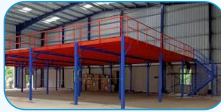
Modular Mezzanine Floor
