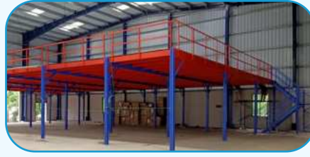
Modular Mezzanine Floor
