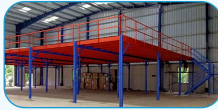
Modular Mezzanine Floor
