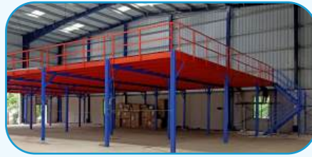
Modular Mezzanine Floor
