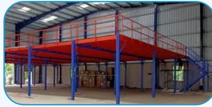
Modular Mezzanine Floor
