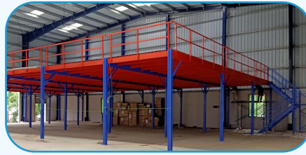
Modular Mezzanine Floor
