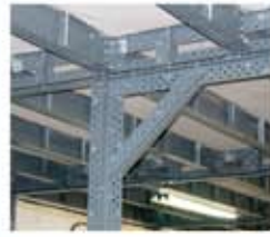
Slotted Angle Mazzanine
